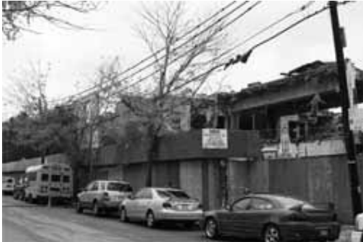
Demolition work is underway for the site that will house a 13-story building with a three-story mall. PRESS Photo by Ira Cohen
